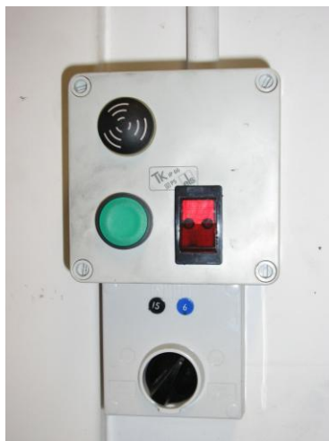
Figure 3. Door pulley controller
