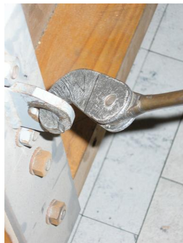
Figure 4. Pulley cable hook attachment to chamber door.
