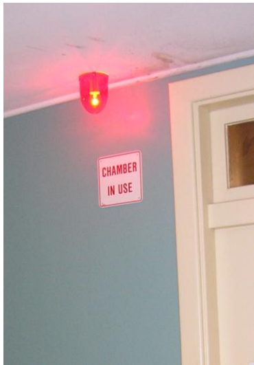
Figure 5. Chamber door closed indicator.
